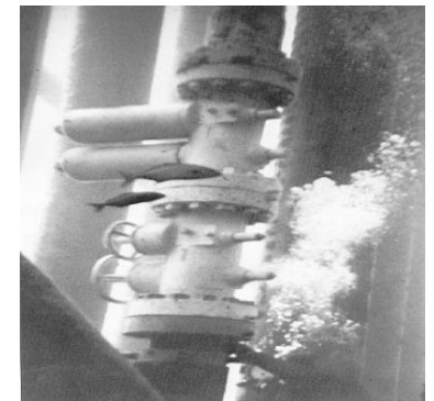
Fire Safe Valves Under Platform 1968
